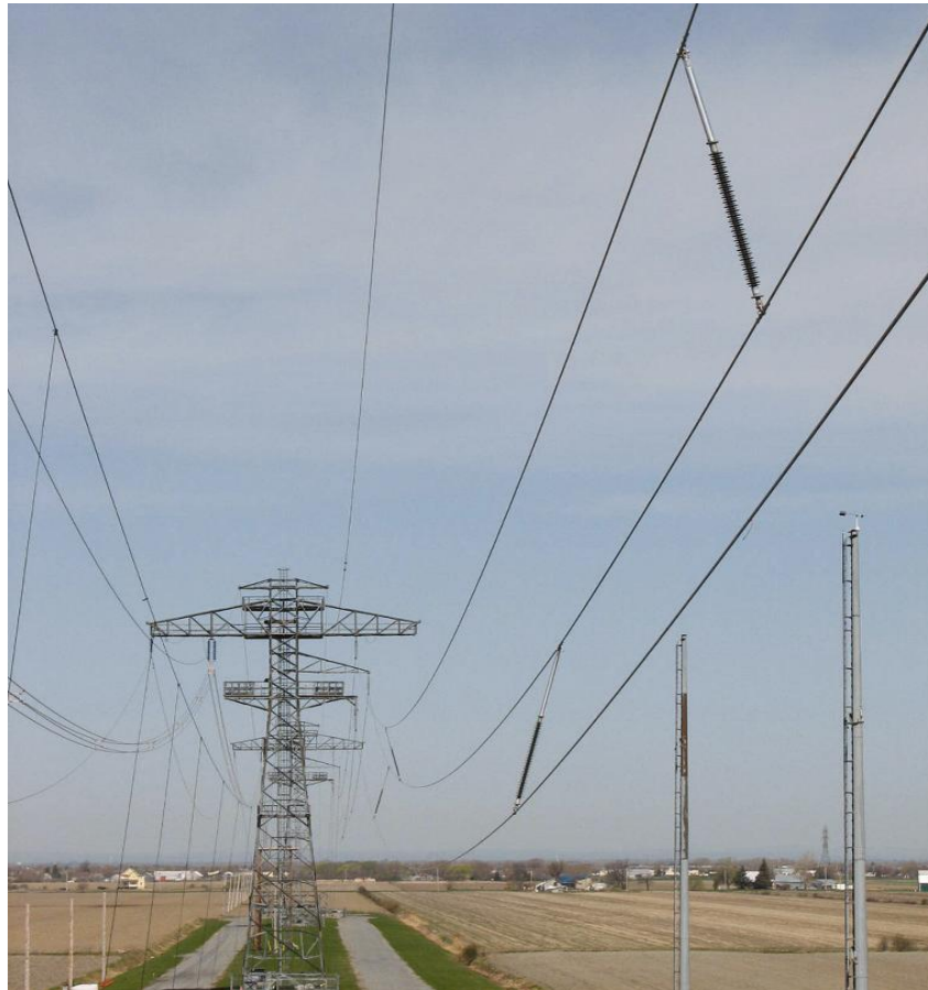
Figure 21: Interphase spacers on transmission line [3]
