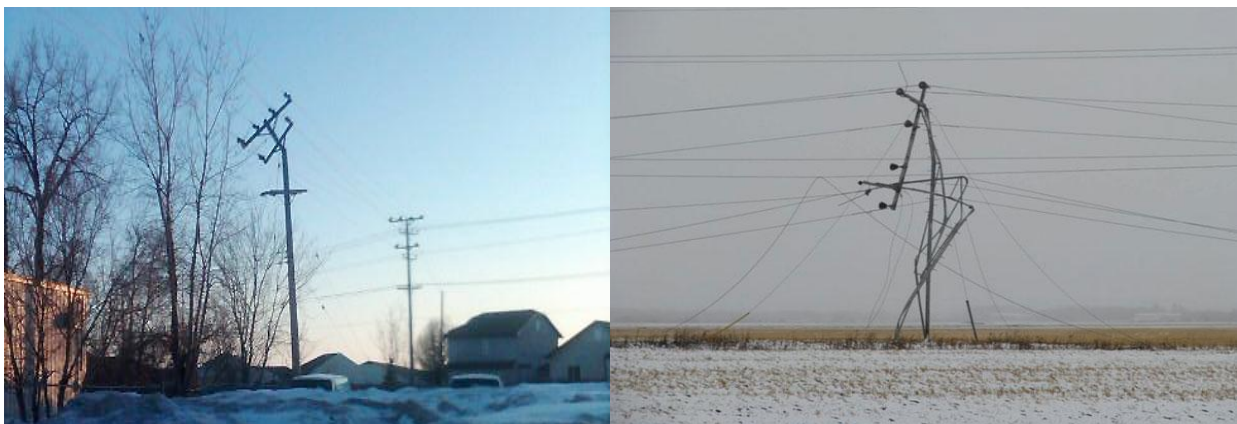
Figure 1: Pole damage and pole fire in L-side and tower bend due to galloping in R-side [2]
