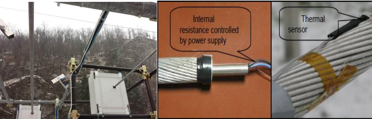
Figure 25: ACSR Conductors Subjected to Slow Rotation (L-Side) and Measure the thickness of Snow Sleeve. ACSR Conductors Intended for the Simulation of AI Current (R-Side)[12]
