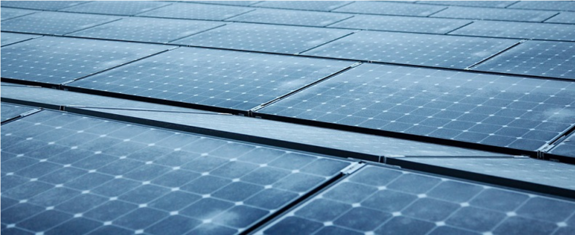
Figure 5.15: Part of the Powerhouse Kjørbo PV system, photo: Sigurd Øygarden Flæten
