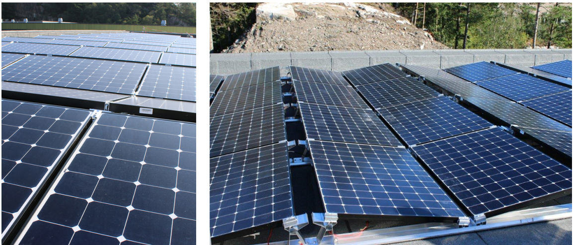
Figure 5.1: Part of the system at Haakonservern shortly after it's installation, photos: Arild Lunde
