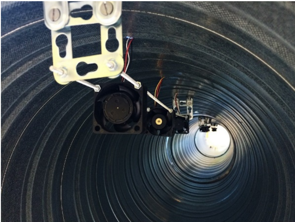
Figure 5: Photograph showing the inside of the experimental model and how the PC fans are mounted
