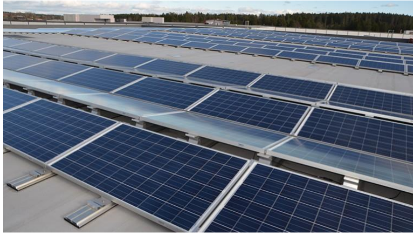
Figure 3. East-west facing rows of PV modules with low tilt angle on one of Norway's largest PV systems at ASKO Øst in Vestby. Photo: Jan Erik Røine/Norsk VVS (used with permission).
