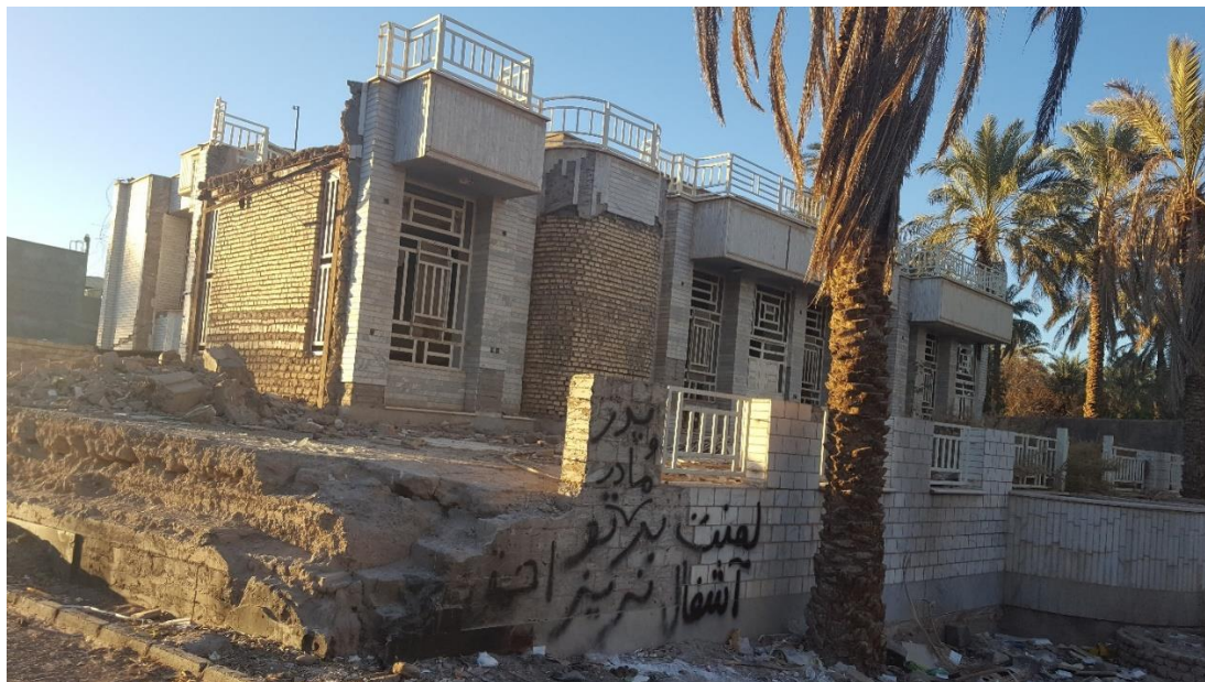
Figure 1. A destructed house remains from the earthquake, Bam, 2018. Photographed by the author.
