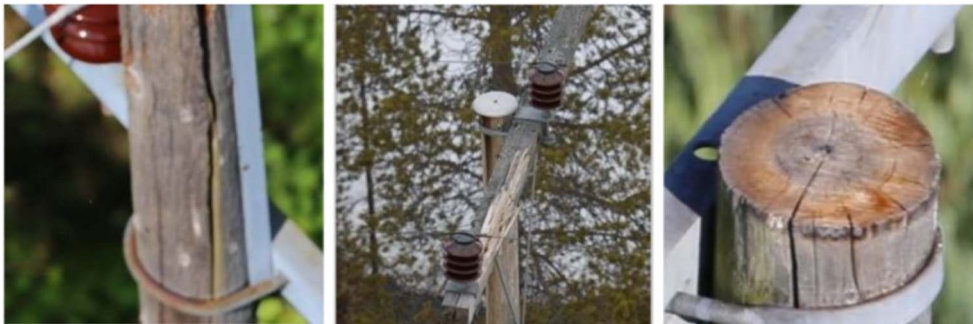
Fig. 2. Common faults on power lines components (from left to right): broken poles, broken crossarms, missing top pads. In Norway, top pads are usually used for protecting wooden poles from rain; thus missing top pads are considered faults. In the US, however, they may not be considered as faults since top pads are not widely applied.
