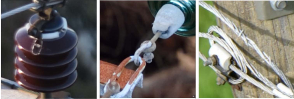
Fig. 6. Small faults on power lines components (from left to right): cracked insulator, missing splint, broken wire.
