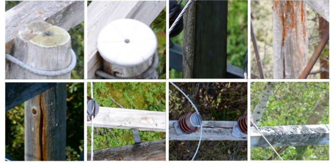
FIGURE 3. Sample images of the DS2_Tc, DS3_Po, and DS4_Cr datasets (from left to right, top to bottom): missing top cap, normal top cap, normal pole, woodpecker-damaged pole, cracked pole, normal cross arm, cracked cross arm, and rot-damaged cross arm.
