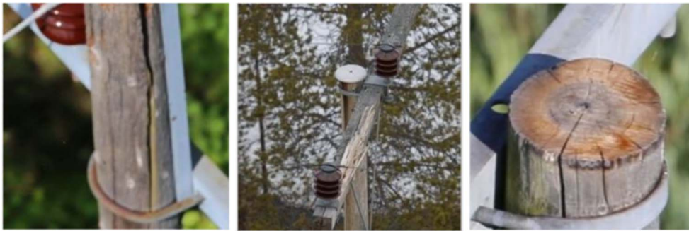
Fig. 2. Common faults on power lines components (from left to right): broken poles, broken crossarms, missing toppads. In Norway, toppads are usually used for protecting wooden poles from rain; thus missing toppads are considered faults. In the US, however, they may not be considered as faults since toppads are not widely applied.
