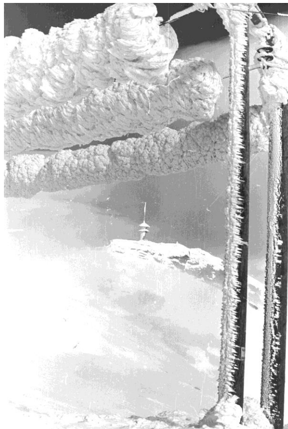
Figure 4 – Lønahorgi ice accretion event in Voss, Hordaland County, Norway, 1961 (photo: Olav Wist). According to Svein Fikke the measured iced diameters were in range of 1.1–1.4 meters with the accumulated ice masses per unit length were in the range of 301–305 kg/m. Figure taken from (IWAIS 2015).
