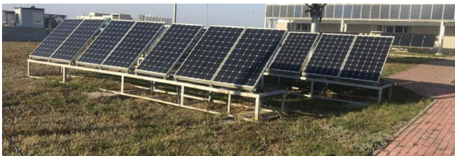
Figure 2. PV solar panels connected to the “Yurt” building
