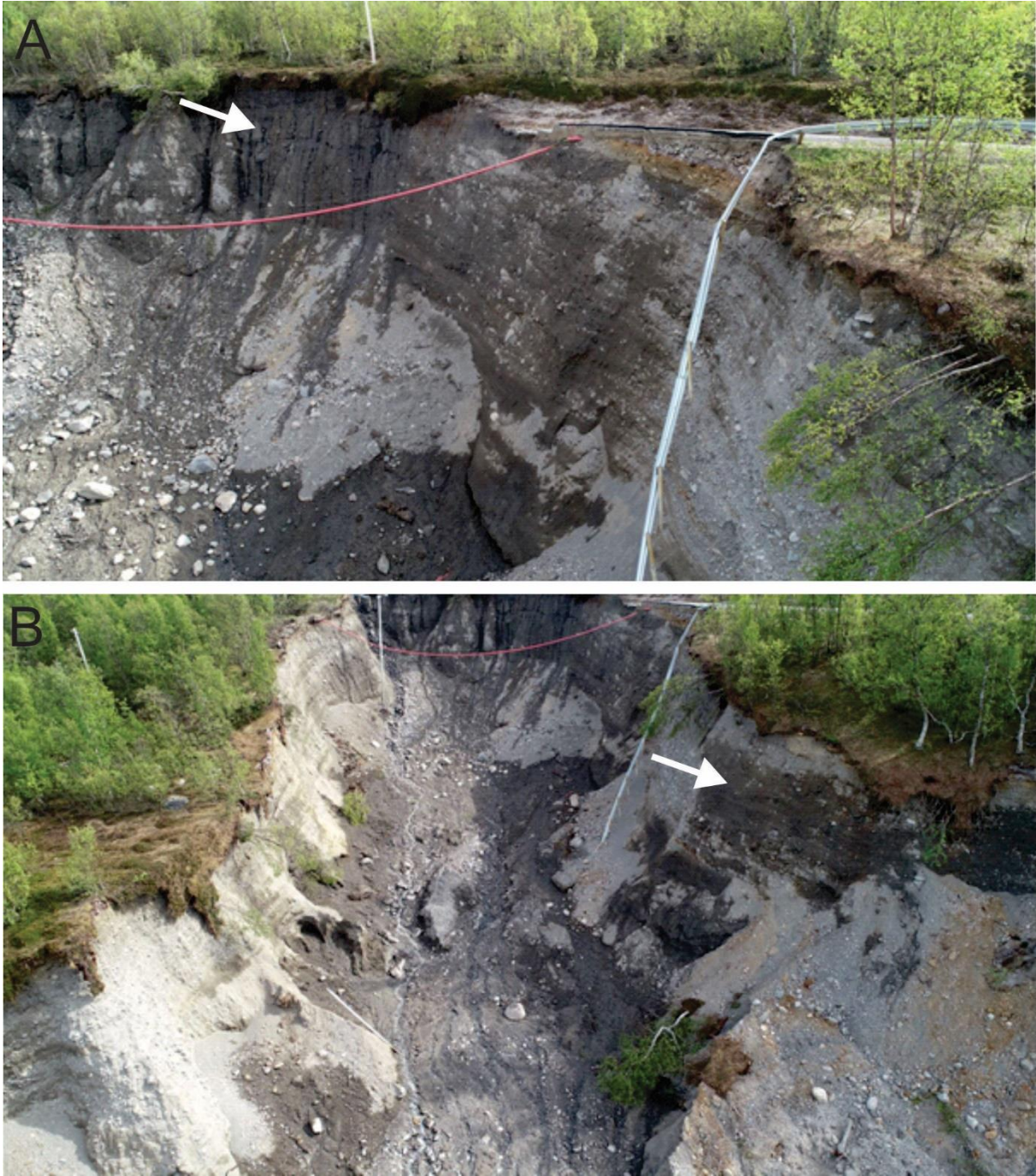
Figure 50 A) Landslide pit and back-scarp up to 40 m asl. Beddings of material 6. The arrow shows water seepage from the back-scarp. B) Braided water streams below the back scarp.
