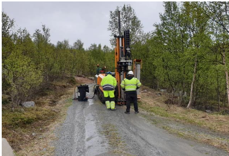
Figure 31 Hydraulic bore rig used to collect bore samples by Multiconsult. Photo courtesy Anders Bjørdal (NVE).
