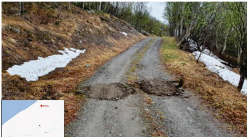
Figure 77 Fracture in the access road to Kråknes Road 450. The fracture is filled with sand. Photo courtesy of Egil Bakkeby (Gylland et al., 2021).
