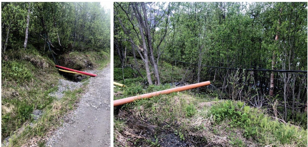
Figure 83 Culverts added to increase drainage to the beach through the tractor road.
