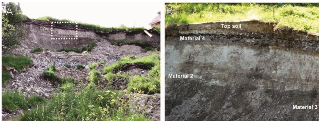
Figure 44 A) Gravel, Material 2 and 3 in the back-scarp of Outcrop 2. B) Close-up of the dashed square in A.
