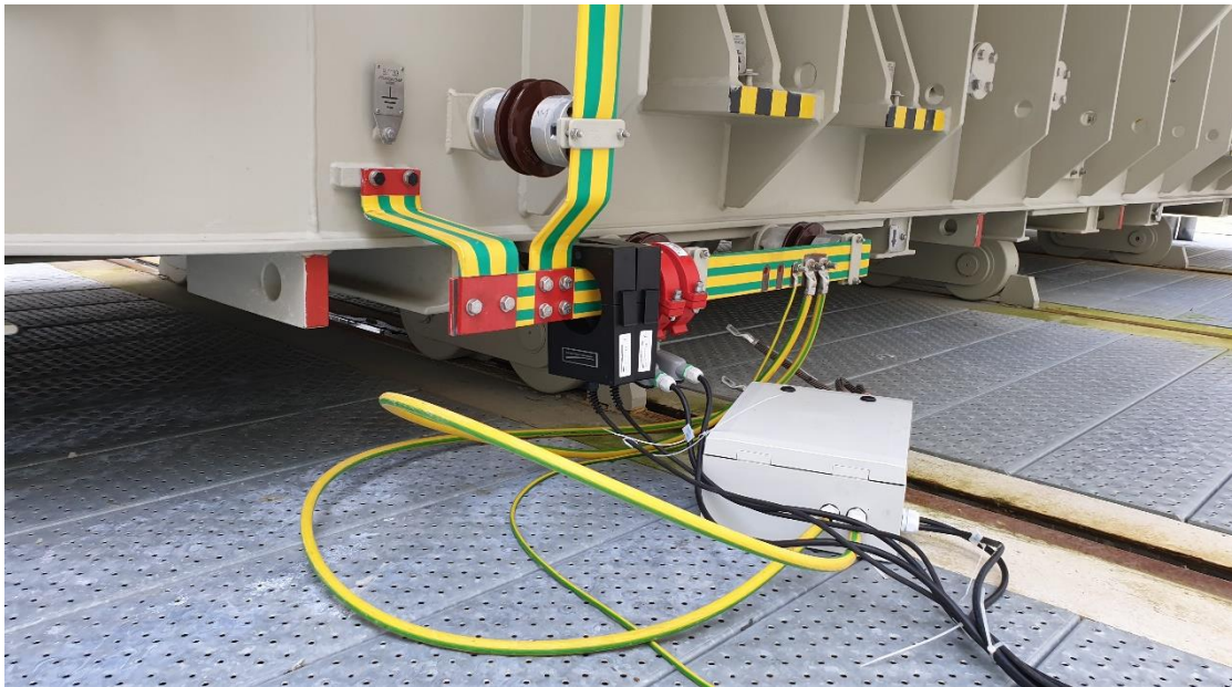
Figure 3-1: Four GIC-sensors (2 black and 2 red) on transformer neutral. Regular hall effect sensor in grey box, see Figure 3-2.
