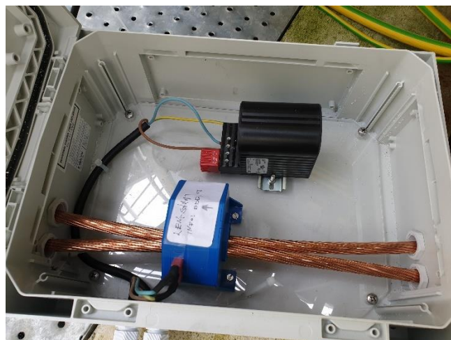
Figure 3-2: Neutral of transformer thread through a regular hall effect sensor (blue). Also a heater (black).
