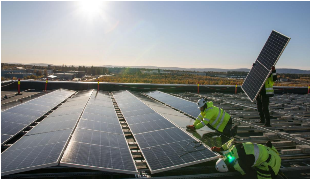
Figure 1: East- west orientated PV system with an annual power production of 2,85 GWh installed on the roof of Coops main warehouse in Jessheim, Norway (Teknisk Ukeblad, 2021).
