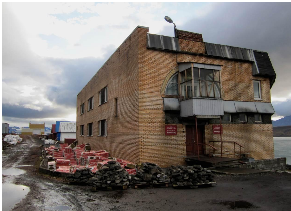
Figure 5. Keeping continuity in Arctic expertise, renovation work in the summer of 2011 on the research station of the Russian Academy of Science in Barentsburg, Svalbard. Photo: Urban Wråkberg.
