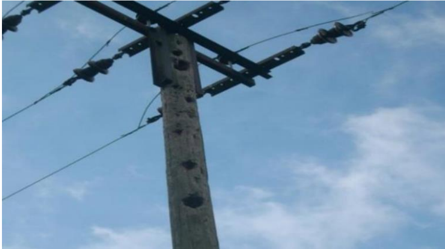
Figure 10: Wooden pole with several holes from woodpeckers.
