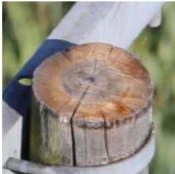
Figure 11: Example of wooden pole missing top pad.
