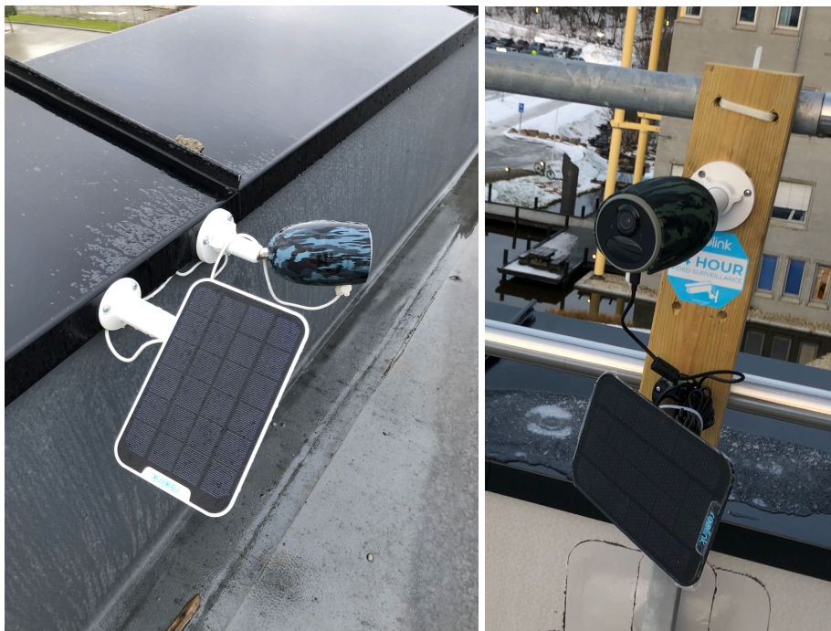
Fig. 60. Cameras mounted adjacent to the OES and ILP systems.
