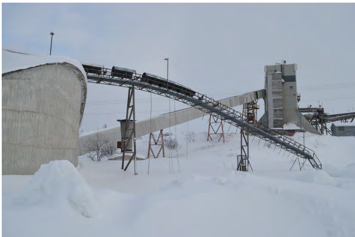
Figure 7: Degrading conveyor belt into the storage silo. Peeling metal siding of the rock crusher building is visible in the background (photo by Anatolijs Venovcevs).
