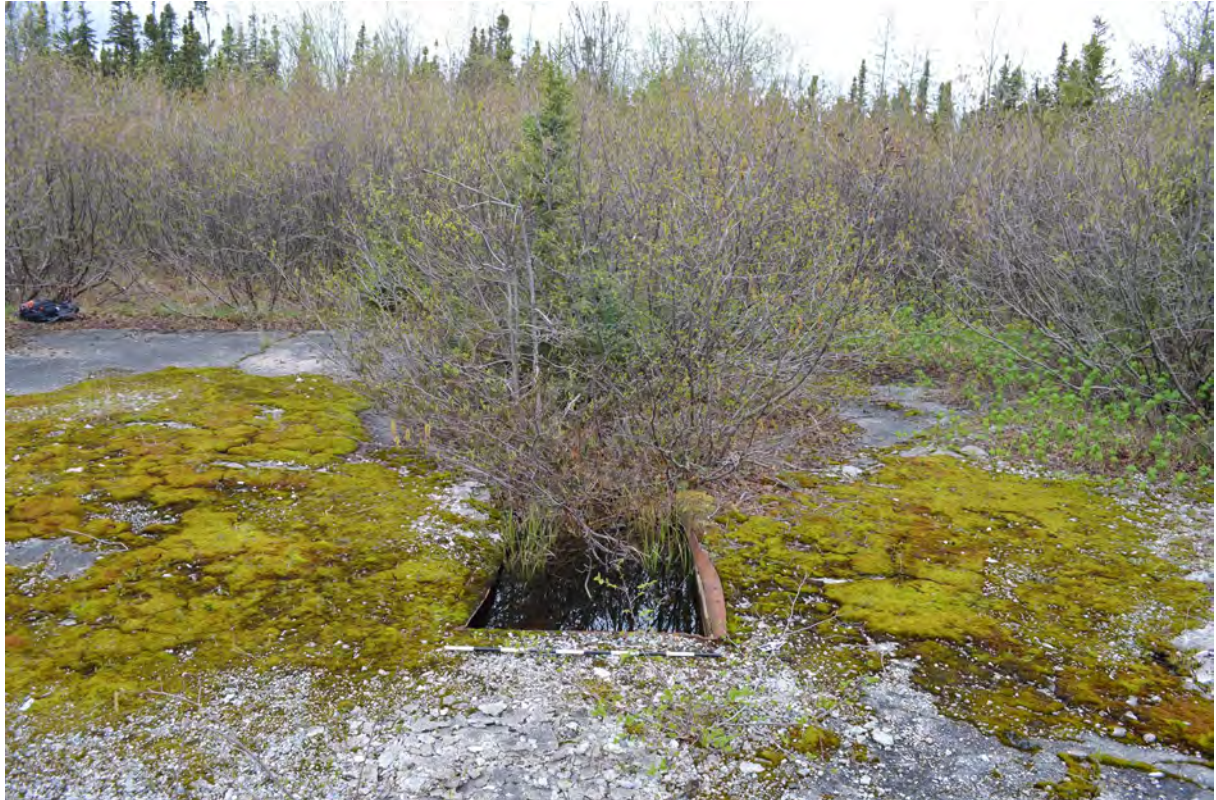
Figure 29: Service pit in the former garage at Twin Falls with a meter stick in front of it, June 10, 2021.
