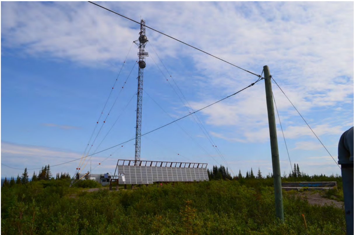
Figure 56: Cell phone tower outside of Labrador City, the foundation of an earlier communications tower is visible on the right, August 18, 2019.
