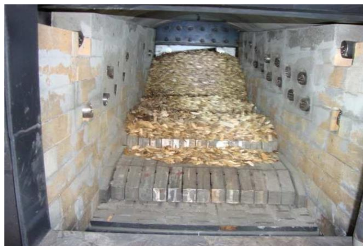
Figure 10. Biomass wood chips on the moving floor
