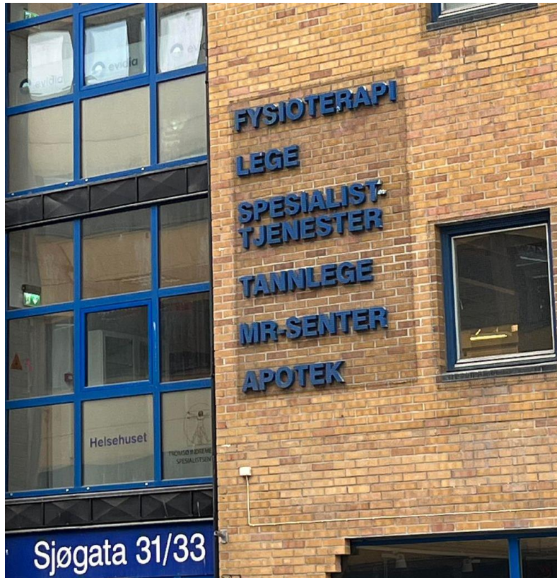
Figure 6: Netting over wall signage at Sjøgata 31/33 in Tromsø (photographed by author).
