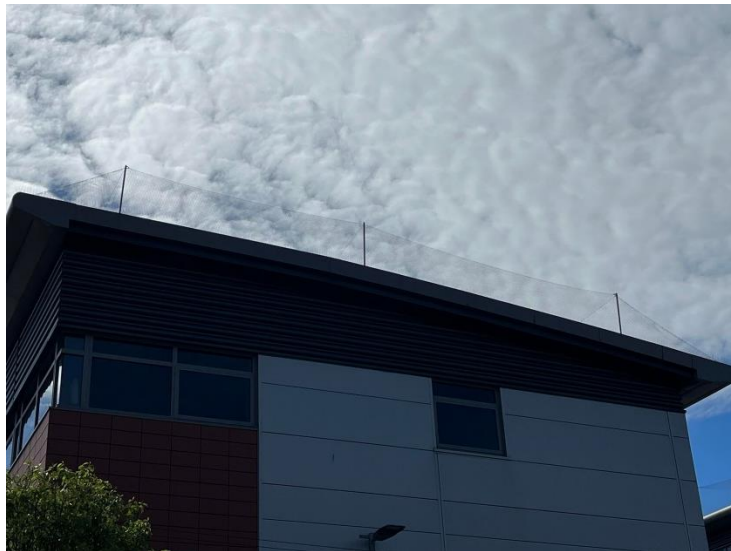
Figure 11: Roof netting on Sanctuary Care building in Worcester (photographed by author).
