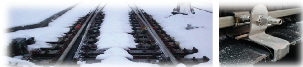
Figure 1. Railway switch operation in icing conditions and location of heater [2].
