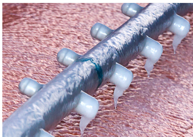
Fig. 20. The Palfinger FF1200 lifeboat sprinkler nozzles before deicing (Sundsbø and Jacobsen, 2018).
