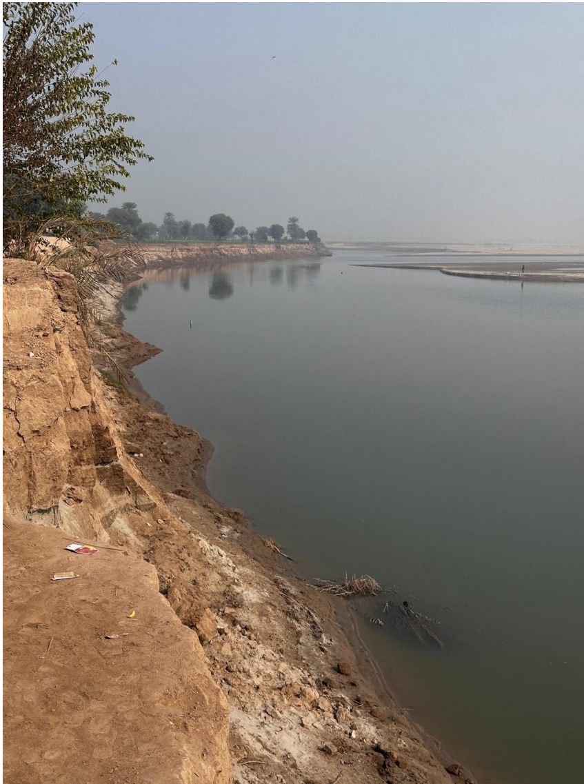
Fig. 4.1 shows the soil erosion on the bank of Chenab river after 2022 floods near Village Marrian, Punjab
