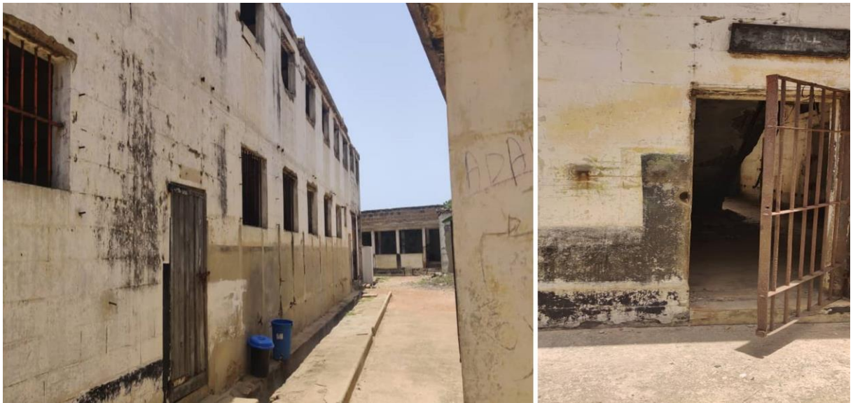
Figure 11: Image Showing a Lack of Maintenance Inside the Usher Fort Prison (Source: John Keney Ademang).
