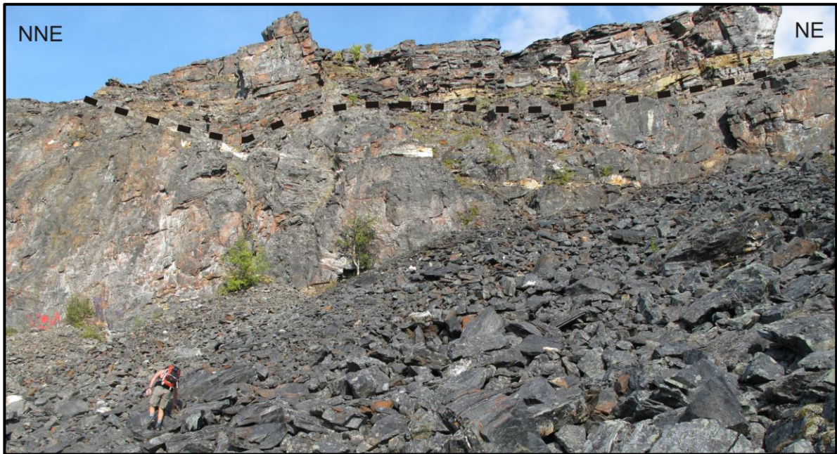
Figure 3.5: The photo shows a lithological contact between the more competent amphibolite and the fractured hornblende schist. Notice that the bedrock in the upper part of the scarp displays a more fractured appearance than the lower amphibolites. Photo is taken looking up from the talus area in the north of the RSF area.
