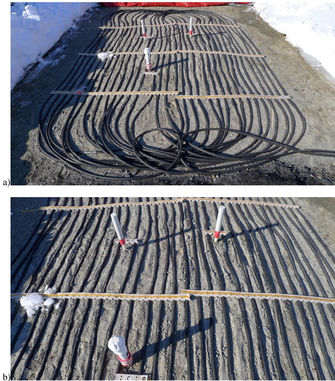
Fig. 1. (a) Overview; (b) close-up of hot-water pipes laid out on gravelly sand, April 19th, 2012 (images by Svein-Erik Sveen)
