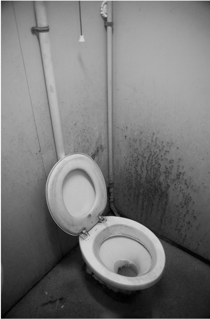
Picture 13: Degrating facilities, such as dirty and dysfunctional toilets, are common at the UPPs. This is an example of one of the better toilets.
