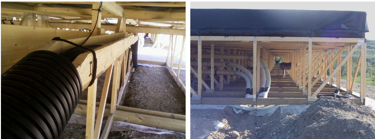
Figure E.35: Between sections of the HBA array, the cables are routed underground. Perforated drain pipes provide a deterrent against rodents. Likewise, at the point where the cables leave the array area to go to the cable mausoleum, they are routed through perforated ducts (right) which go underground.
