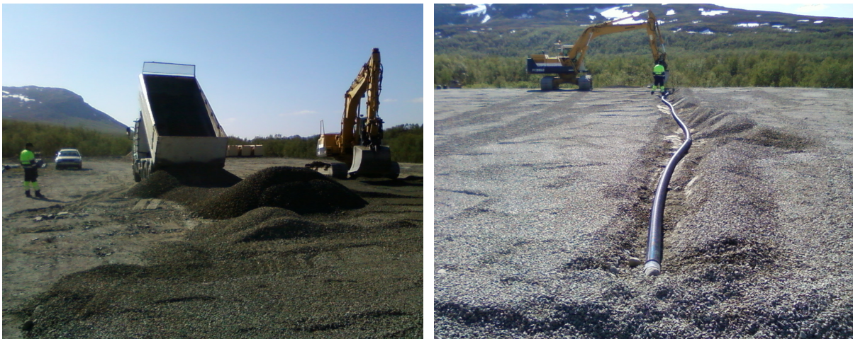
Figure E.15: Gravel being applied for the HBA array drain layer (left) and an example of the embedded perforated drainage pipes (right).
