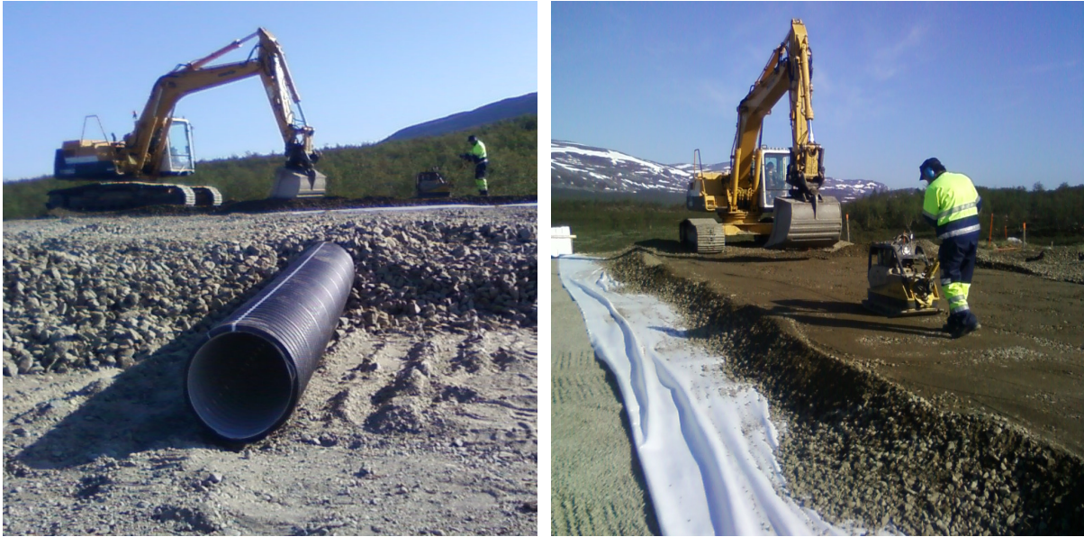
Figure E.16: Left: Side view of the drain layer with protruding drainage pipe. Right: application of the final gravel layer over geotextile.
