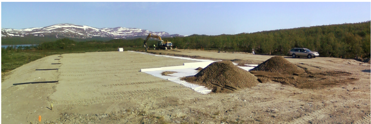
Figure E.18: North-northwest facing composite image of the site, showing the final gravel level being applied over the geotextile. The intermediate layer can be seen in the centre and left, with the drain pipes protruding from this layer on the left.
