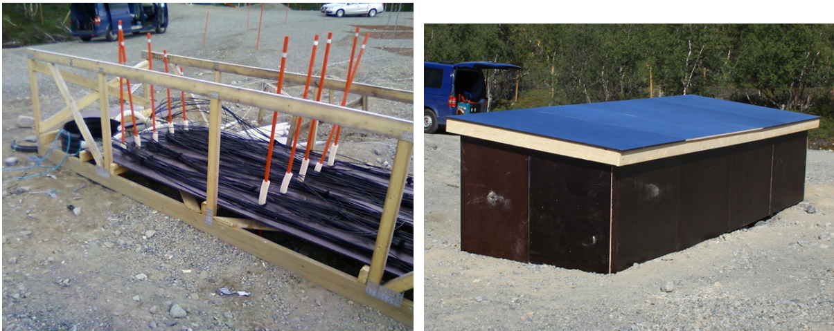
Figure E.44: The LBA cable mausoleum during construction (left) and after completion. The cables zig-zag back and forth without any loops, before going into the subterranean main duct (the large black entry point to the left). Compare the LBA cable mausoleum to the HBA cable mausoleum (shown in Figure E.36).
