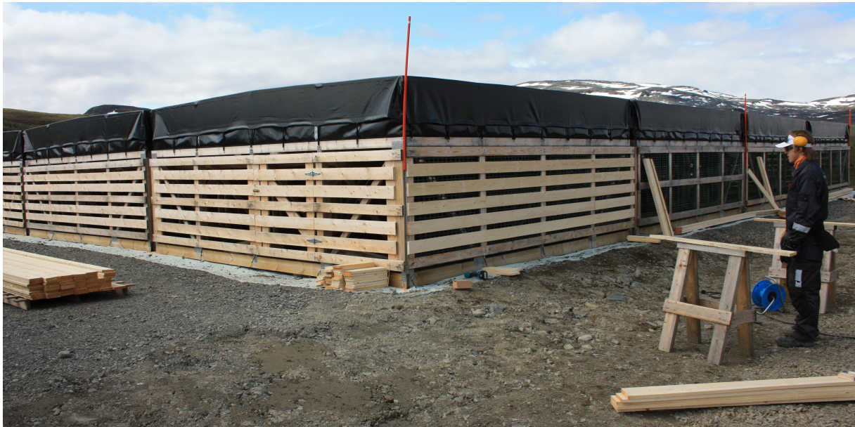
Figure E.37: Application of the snow panelling and mesh on the sides of the HBA framesets. The panelling included several doors, to permit access to the underside of the array. The panels not only prevent excessive snow drift under the array, but also exclude large wildlife (c.f. Figure E.35, right). Image: Arttu Jutila, SGO.
