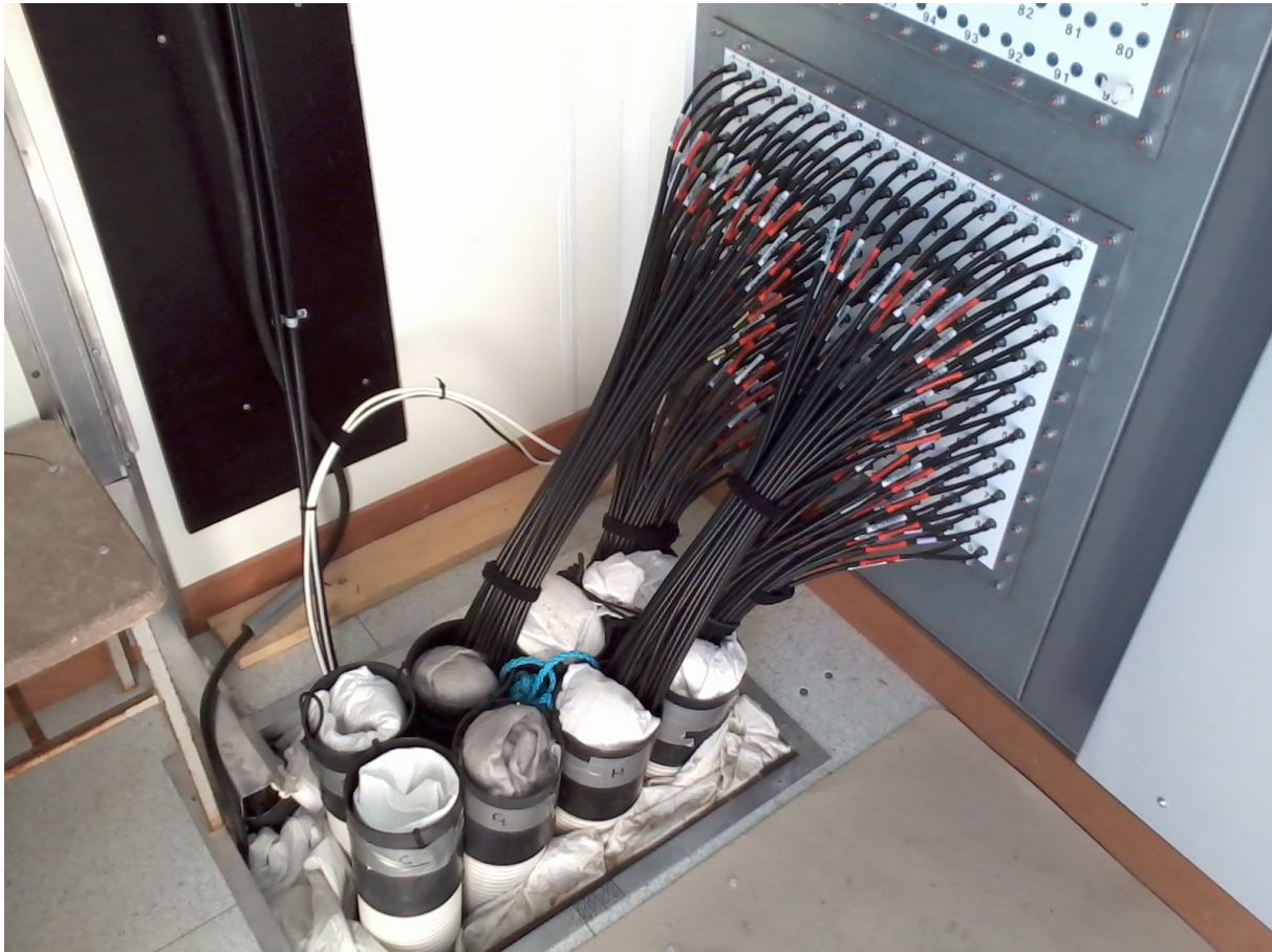
Figure E.50: Just inside the electronics cabin is an RF-tight patch-panel, which interfaces cables going into the Faraday enclosure.
