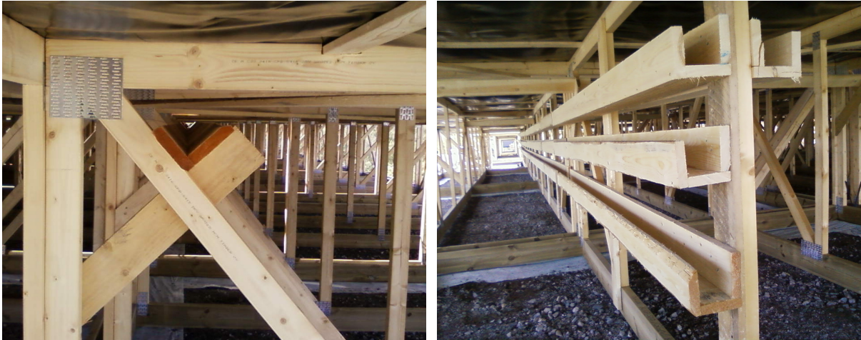
Figure E.34: Left: Example V-section cable tray for each row on HBA tiles (per row: 6 tiles = 12 cables; c.f. Figure E.20). Right: U-section cable trays forming the main trunking. In both cases, the cables are not yet in place. Each U-section tray serves two rows (12 tiles = 24 cables).
