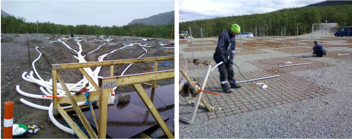
Figure E.43: Digging shallow trenches and adding the cable ducting drain pipe (left) and the feeding of cables into the ducts in the backfilled area, after the RF ground planes had been placed (right).
