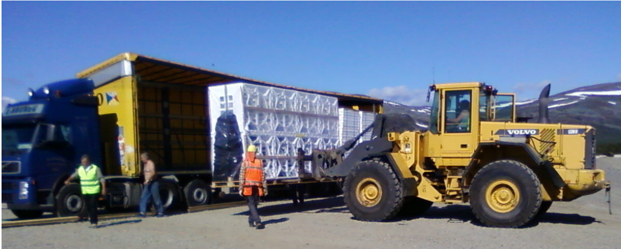
Figure E.24: Unloading the HBA tiles from the delivery lorry. Such a heavy-duty fork-lift vehicle was not required; however it was the only one available. The folded tiles (including packing material) weigh approximately 250 kg.
