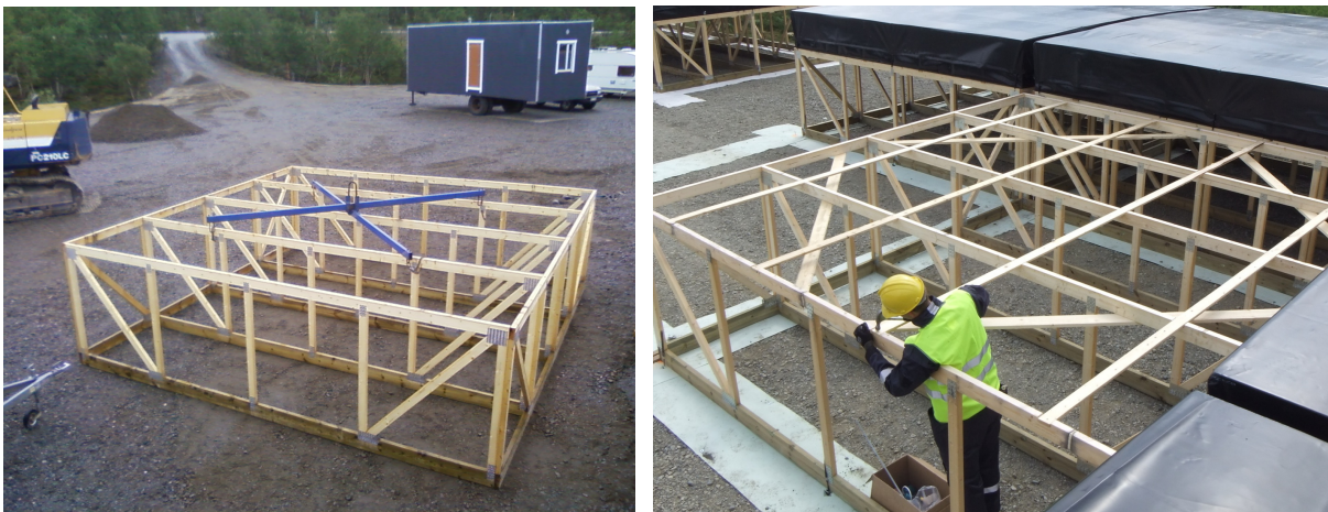
Figure E.21: Left: A completed frameset, prior to being lifted onto the HBA array field. The blue metal hoisting cross is only for lifting the tile into position, and is not part of the final structure. Right: A frameset in position. The additional diagonal braces are being applied. Note the way the frameset sits on the strips of geotextile.
