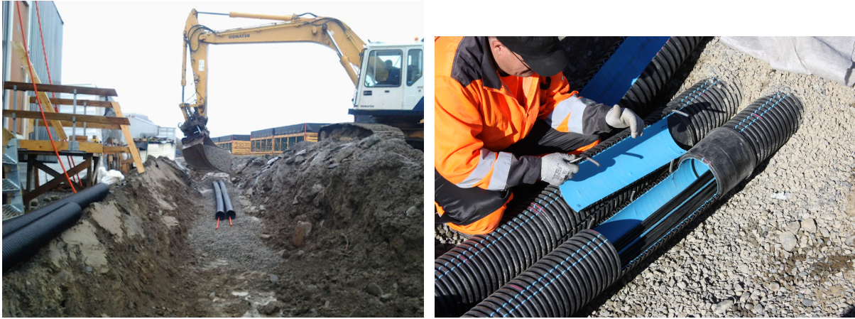
Figure E.45: The LBA main cable trenching with the main ducts being buried (left) and the mid-point access hatches removed (right), showing the cables inside. Photos: Toivo Iinatti & Arttu Jutila, SGO.
