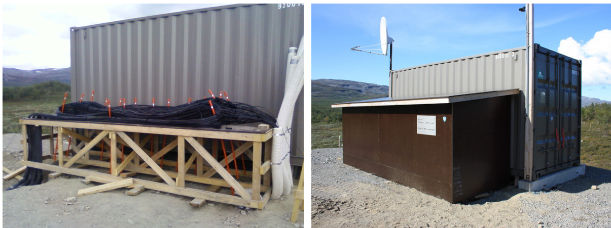
Figure E.36: The HBA cable mausoleum during construction (left) and after completion (right). The grey shipping container is the electronics cabin (RF-container). An LBA mausoleum also exists (see Figure E.44), but it is located adjacent to the LBA array.
