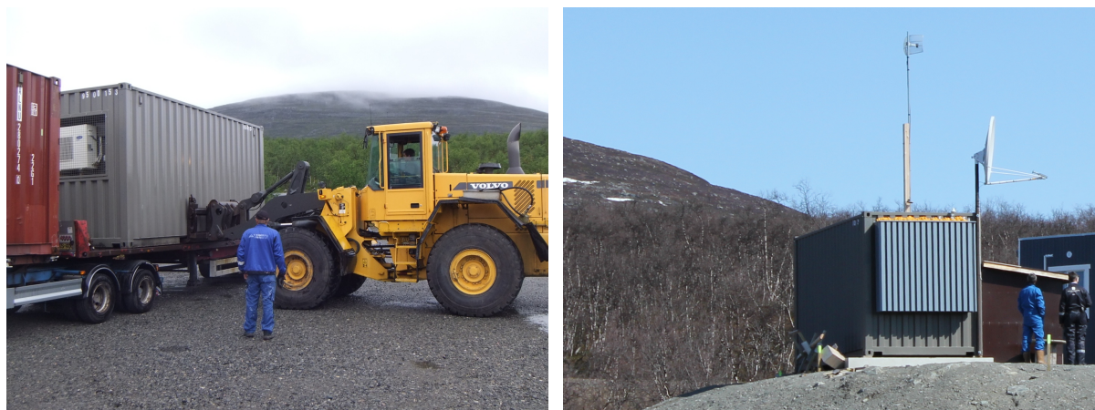
Figure E.49: Unloading the electronics cabin from the delivery lorry. Note the air-conditioning unit embedded in the end of the container (left). The cabin was placed on two concrete foundation blocks (right). After placement, a metal cowl was put over the air-conditioning unit to prevent ice build-up from fouling the radiator fan. See also Figure E.36, which shows the completed electronics cabin.
