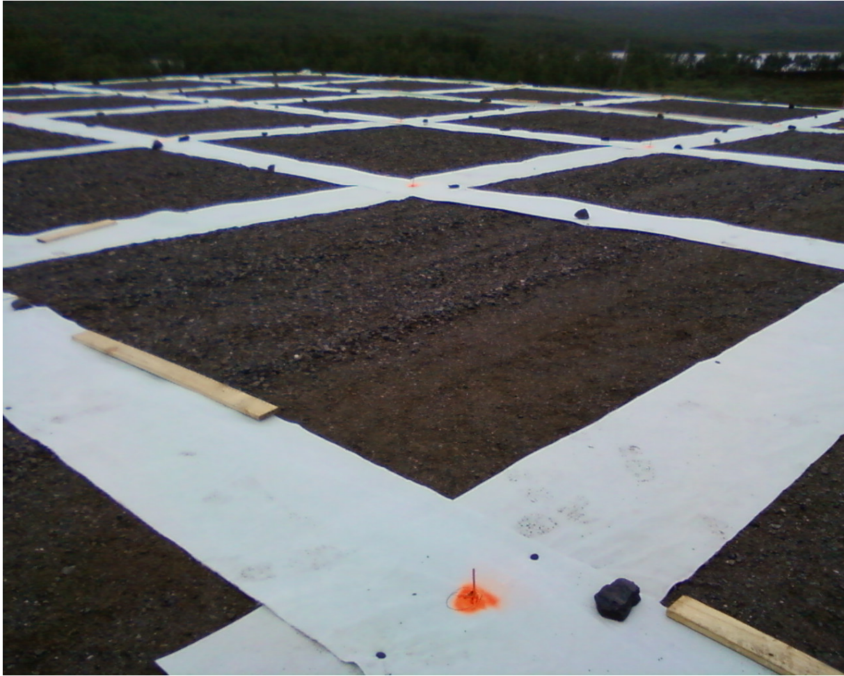
Figure E.19: Geotextile on the HBA array field, placed along the edges where the HBA framesets would be situated. The orange spray-paint dots mark the positions of the steel survey pegs.
