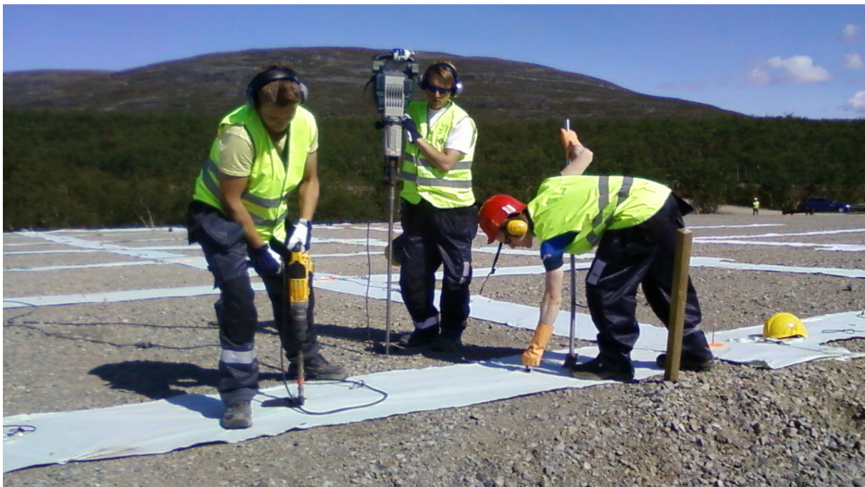
Figure E.22: Anchor lines are installed by first drilling a pilot hole into the ground (left). The duck-bill anchor is placed on the end of an extended jack-hammer bit (centre), and driving into the pilot hole. A lifting rod (right) is then used to provide tension and lock the anchor into place.
