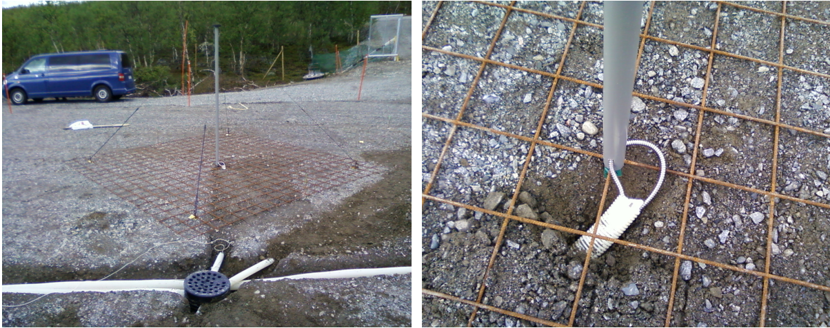
Figure E.46: A newly completed LBA with respect to the cable node and routing pipes (left). The two signal cables are protected with a flexible metal armour at the point where they leave the LBA mast and go into the underground ducts. A wad of geotextile is pressed into each to hold the cables steady and prevent access by rodents.
