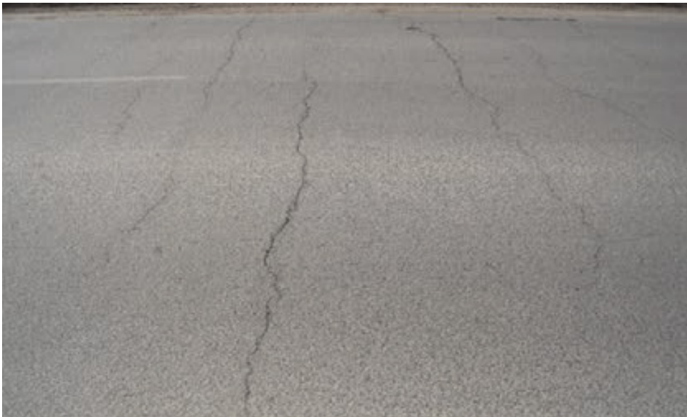
Figure 10: Transverse cracks in the asphalt pavement.
