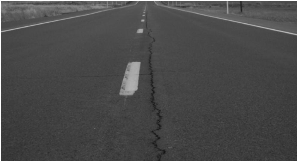
Figure 8: Longitudinal cracks in the asphalt pavement.
