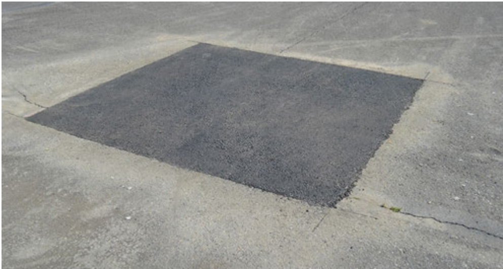
Figure 11: Patch on the asphalt pavement.
