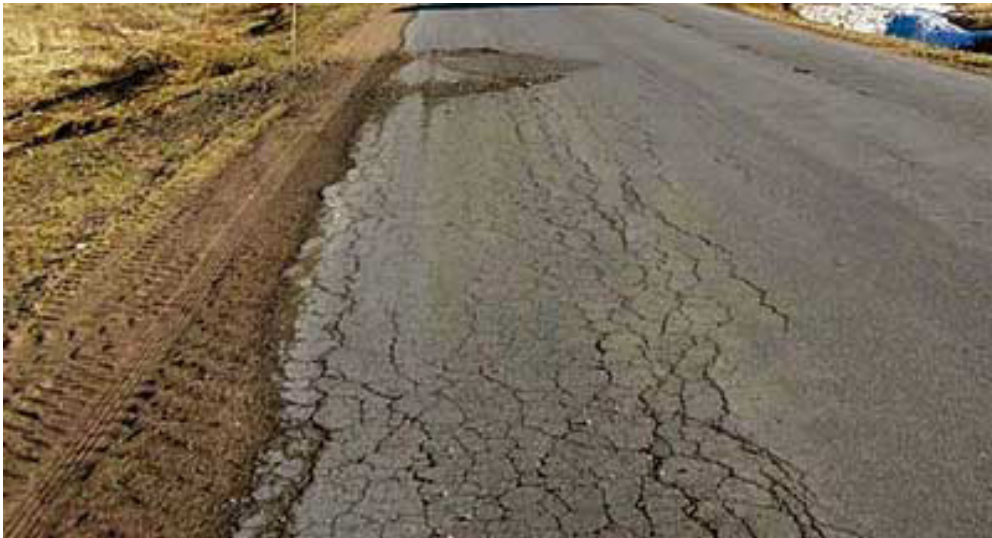
Figure 7: Edge cracks in the asphalt pavement [44].
