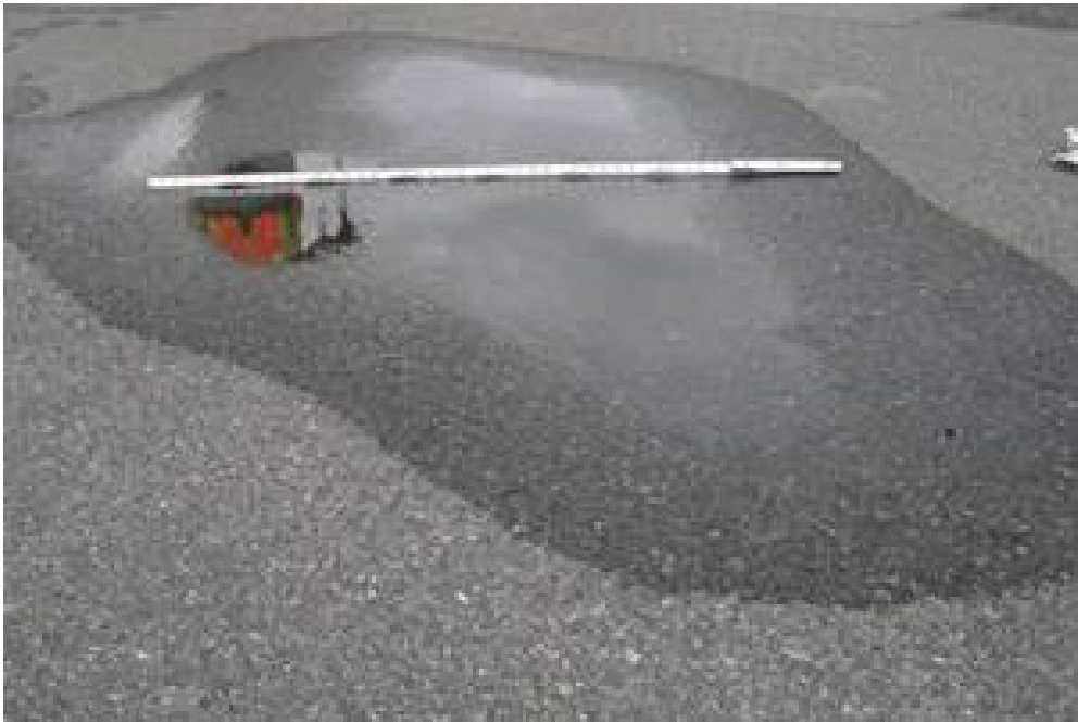
Figure 16: Depression in the asphalt pavement.
