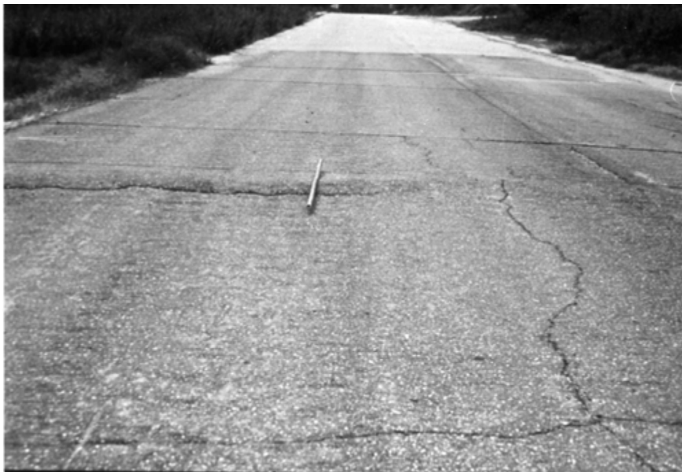
Figure 17: Swells in the asphalt pavement.
