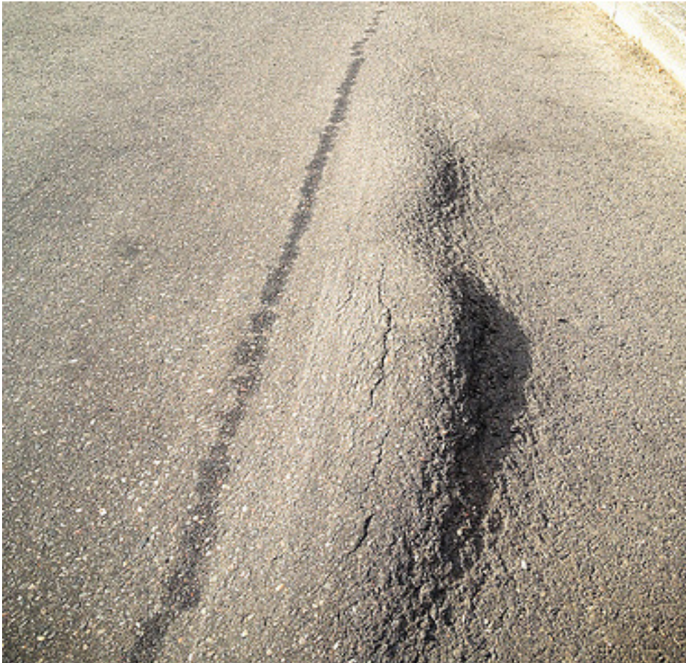
Figure 15: Shoving on the asphalt pavement.
