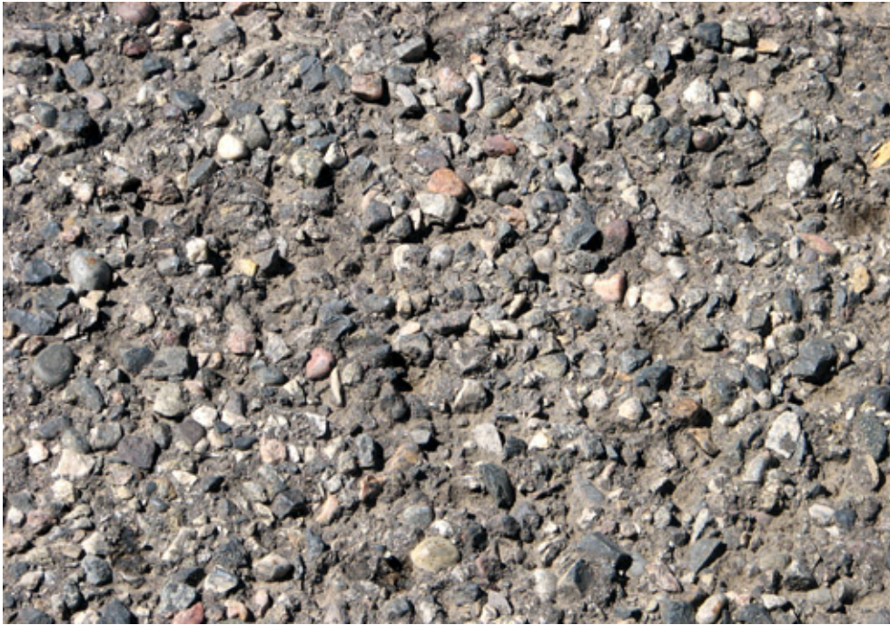
Figure 18: Raveling on the asphalt pavement.
