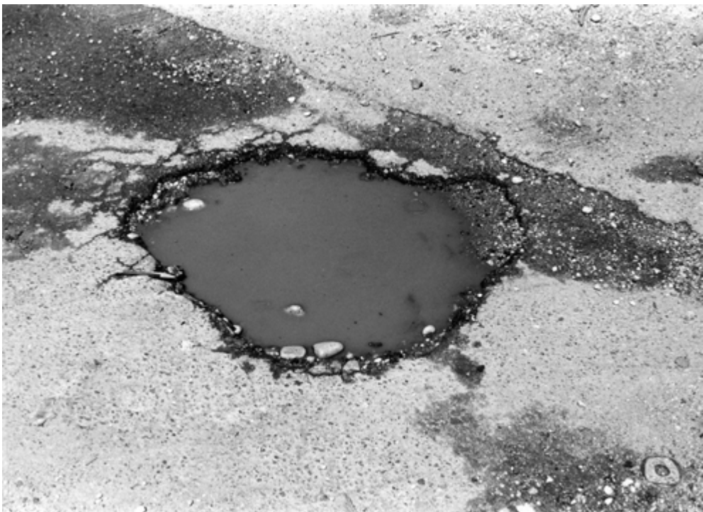
Figure 12: Pothole (filled with water) on an asphalt pavement.
