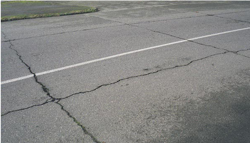
Figure 9: Reflection cracks on the asphalt pavement.
