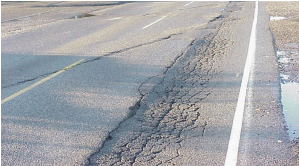
Figure 13: Rutting on the asphalt pavement [45].
