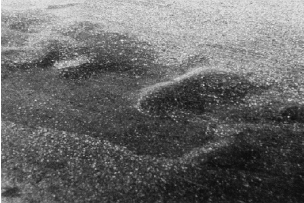
Figure 14: Corrugations on the asphalt pavement [41].
