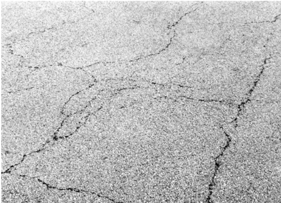
Figure 6: Block cracks in the asphalt pavement.
