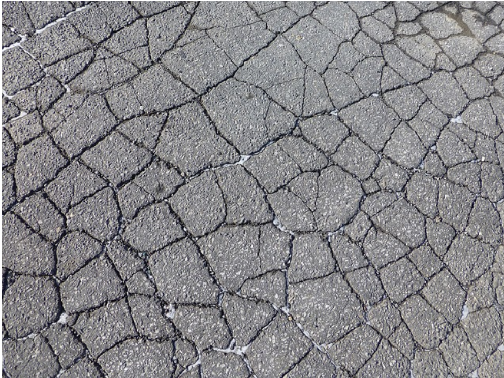
Figure 5: Alligator cracks on the asphalt pavement [42].
