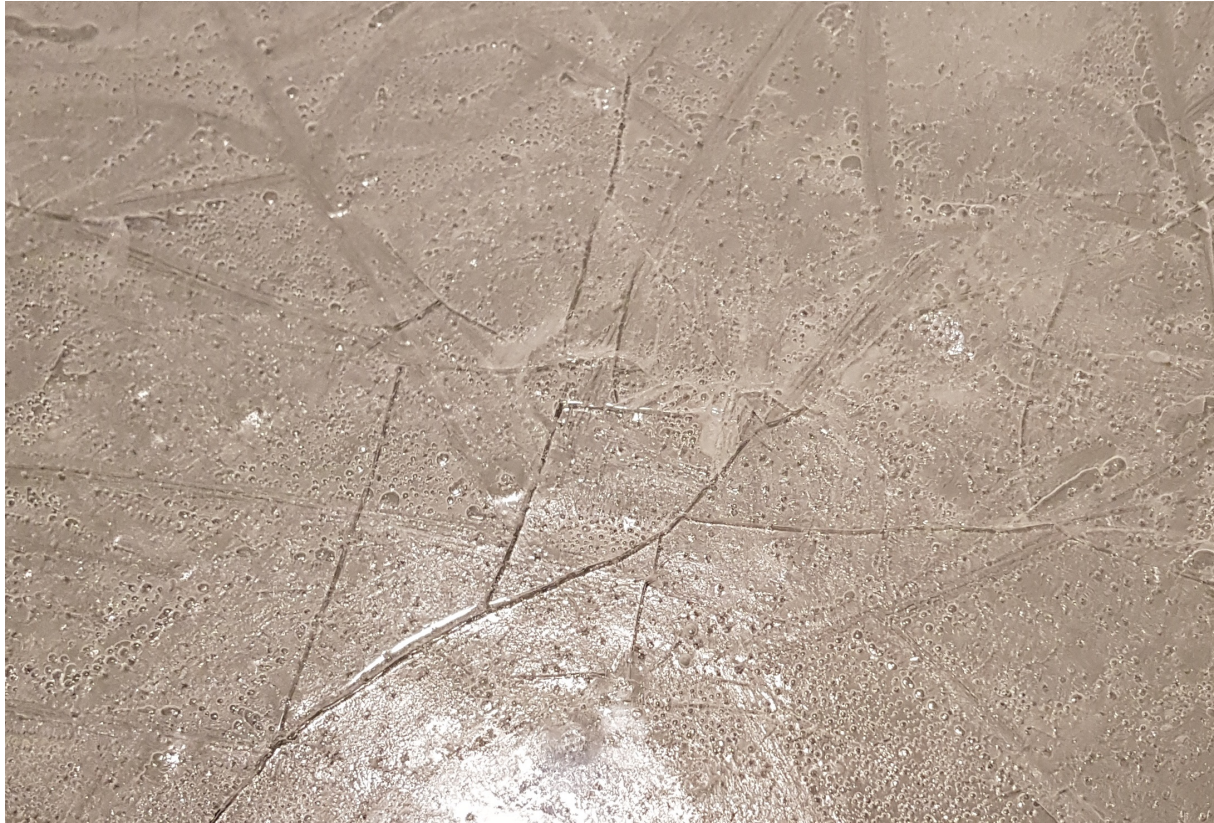
Figure 20: Cracks on polyurethane board with ice
