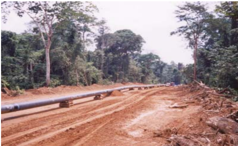
Fig. 3.4. Cleared forests 15 meters on each side of the pipeline. N.B. Picture by Courtesy of Forest People Programme. 167
