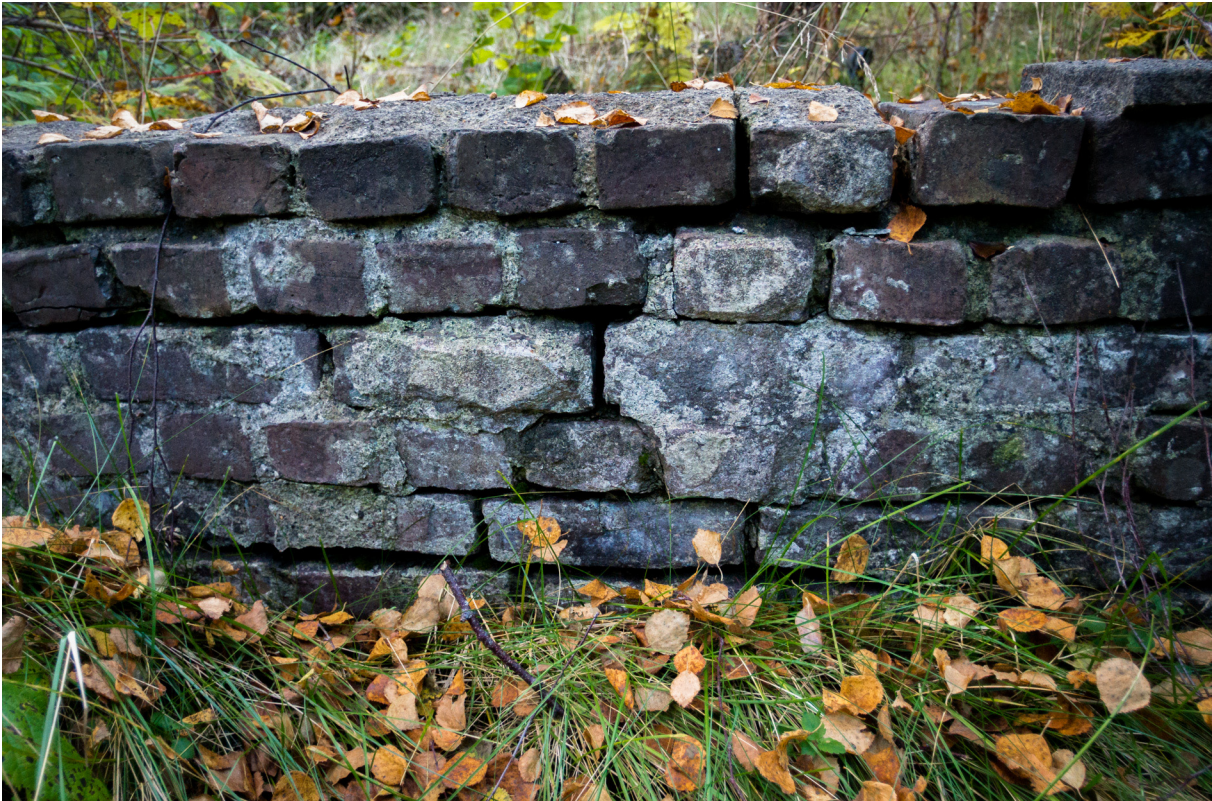
Figure 17 The crumbling pond-wall. The bricks are much more obstinate compared to the malleable and crumbling mortar. 16.10.2015, 16:10.
