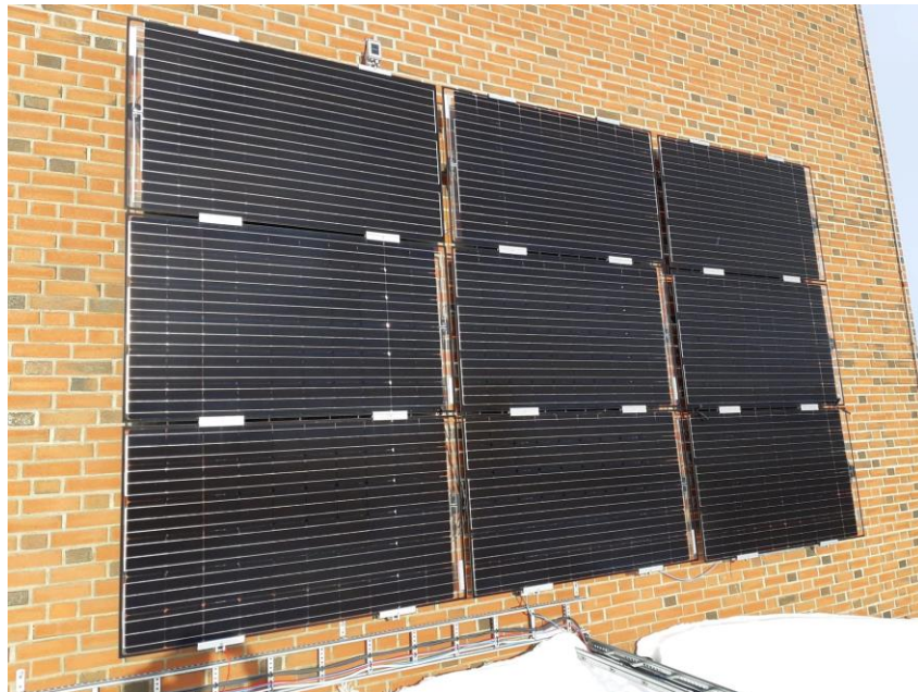
Figure 3-5: Solar modules mounted on facade. Module to the left is non- bifacial, while the other two is bifacial modules. Photo by Odin Foldvik Eikeland
