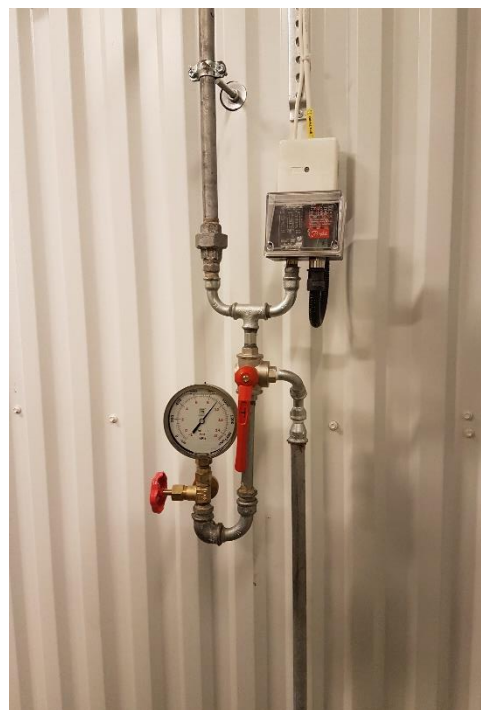
Figur 6. feil kobling, testrør for sprinkler
