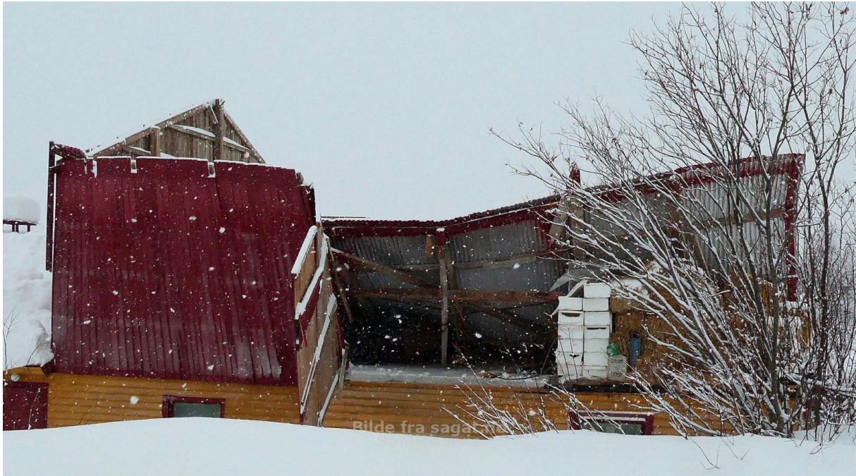
Figure 10: Collapsed barn in Karasjok, northern Norway (Svala, 2020)
