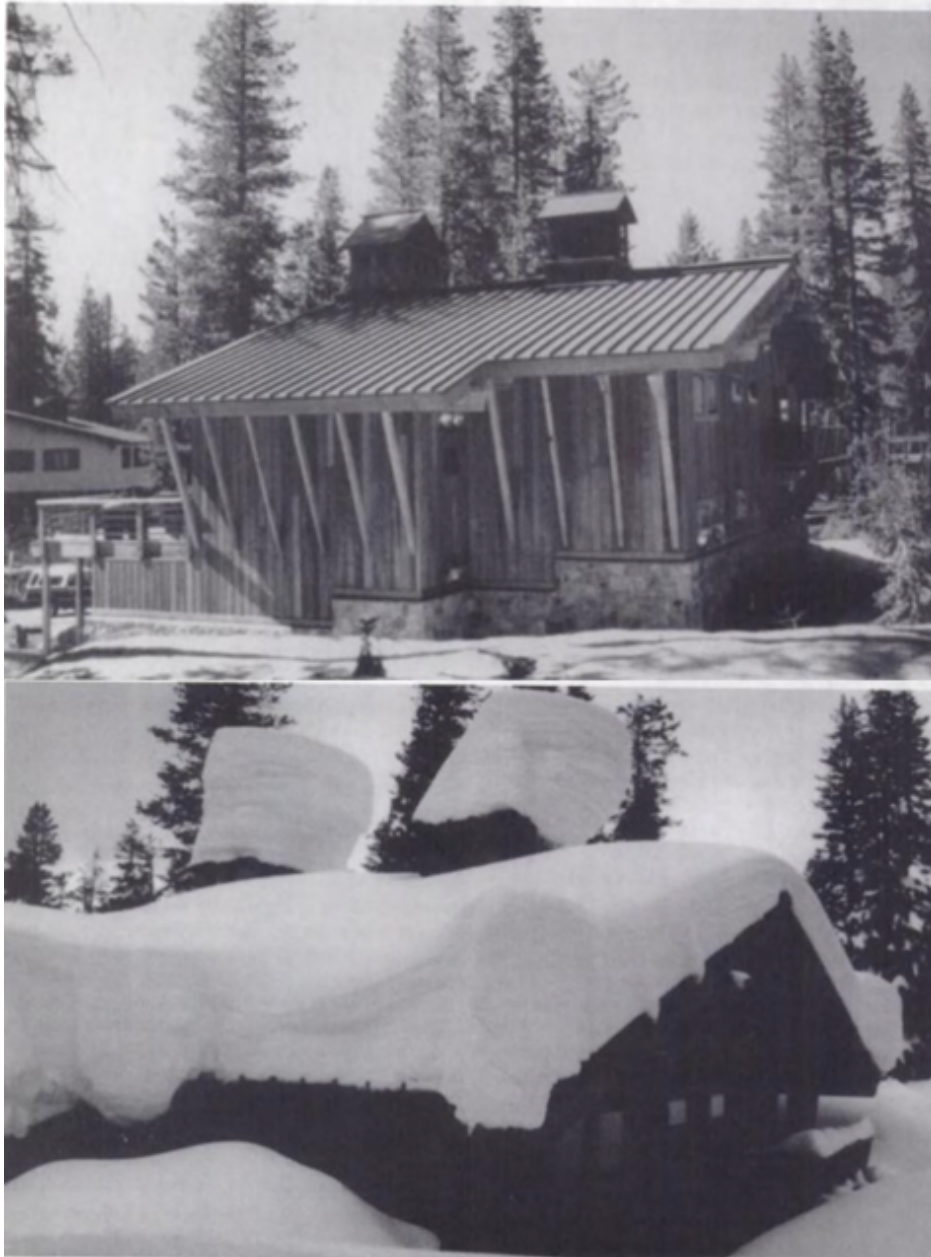
Figure 12: Slippery sloped roof failing to slide off snow (Hjorth-Hansen et al., 2000, p. 214)
