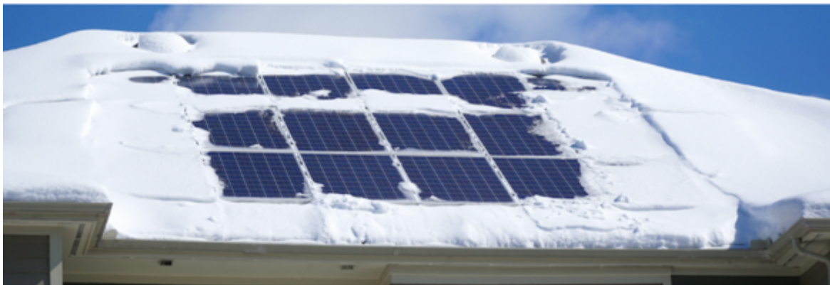
Figure 21: Photovoltaic snow removal for illustration ( www.gocamsolar.com )
