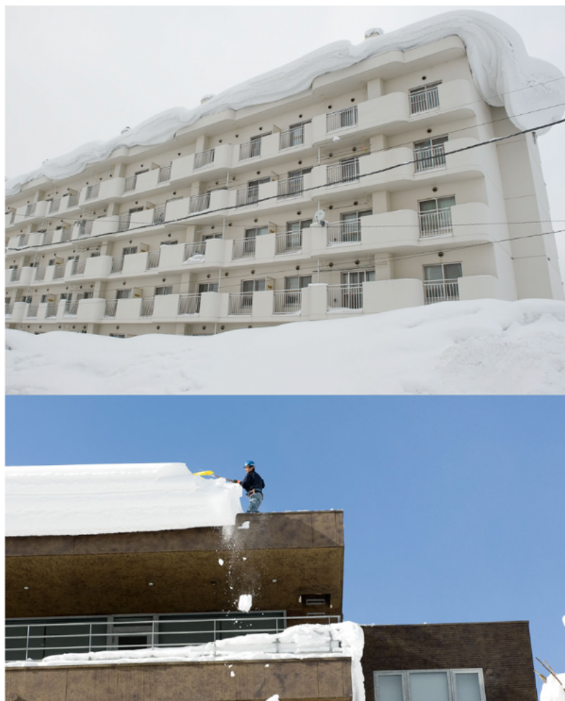
Figure 13: Massive snow cornices at buildings in northern Japan (360niseko.com, 2012)
