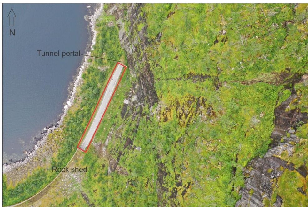
Figure 2. Ortho perspective image of Svarthola, displaying the 100 m long exposed stretch of road (red box) between the tunnel and rock shed. Photo: Linn Asplin, 2020.
