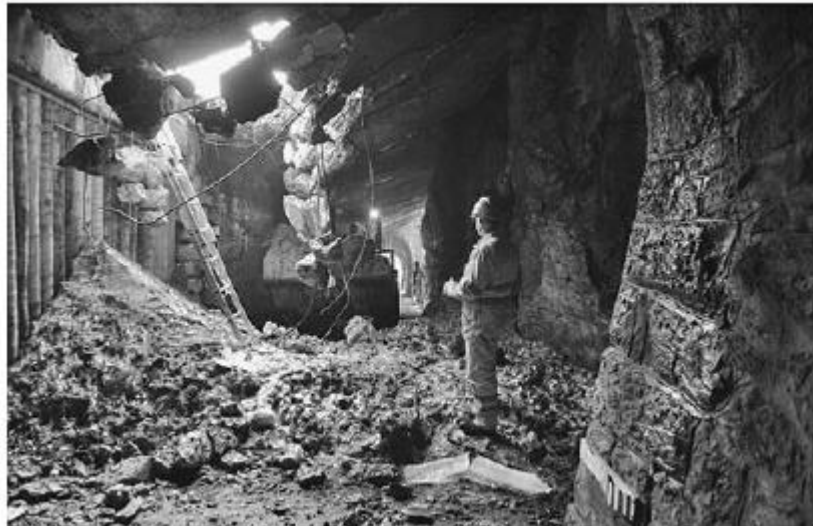
Figure 22. A snow shed that was damaged by a wet-snow avalanche that fell almost vertically on the roof in Switzerland. Photo: Stefan Margreth, 2009.
