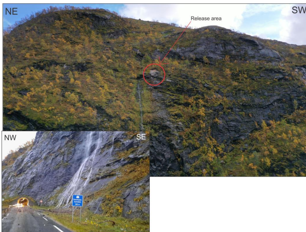
Figure 12. Rockfall event on the 22.08.20. Note the release area (red circle) with fresh exposed bedrock. The estimated volume of the event was less than 1 m 3 , together with loose material. The event closed the road for 13 days due to the work of scaling loose rocks from the slope to prevent further failures (SVV 2020).
