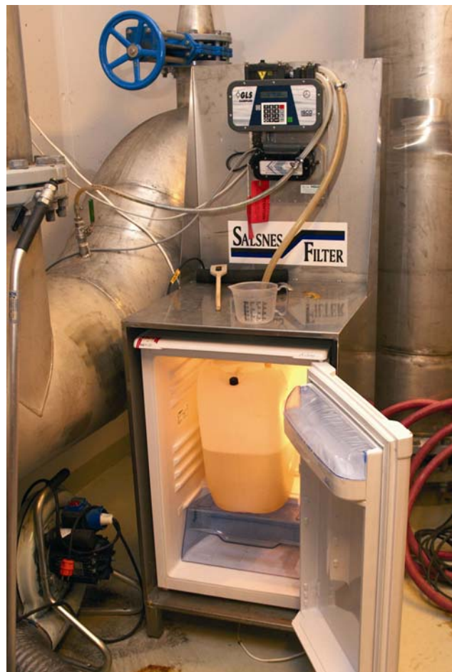
Picture 2: Automatic sampling system of sewage water, Langnes (Tromsø).
