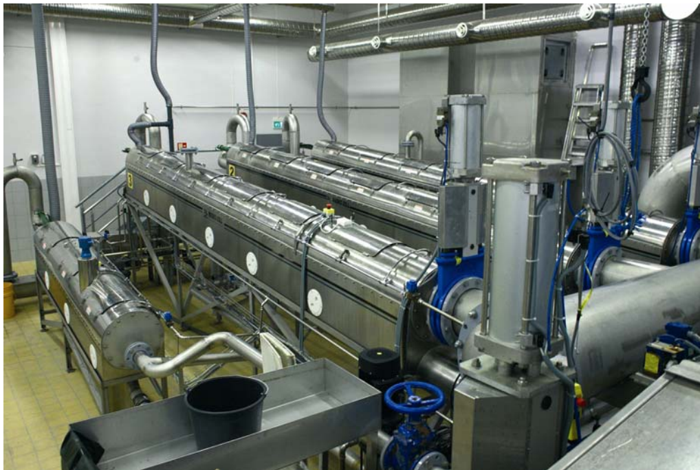
Picture 1: Sewage treatment plant, Langnes, Tromsø
