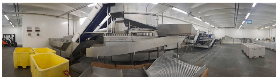
b) Picture showing a processing plant with a single production line. The fish arrive in the plant from bulk loaders at the left-hand side, has the head removed, is gutted, and finally graded into sizes at the right-hand side
