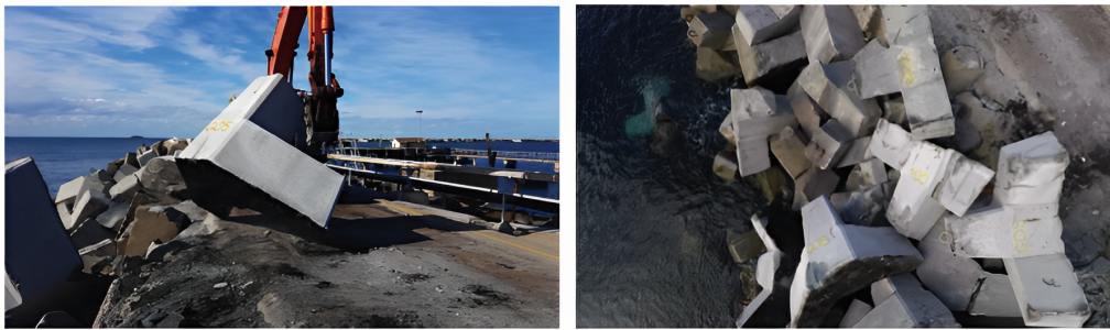
Figure 2.4: Placement of the armour units on the breakwater (left), aerial view of the breakwater (right) [5]
