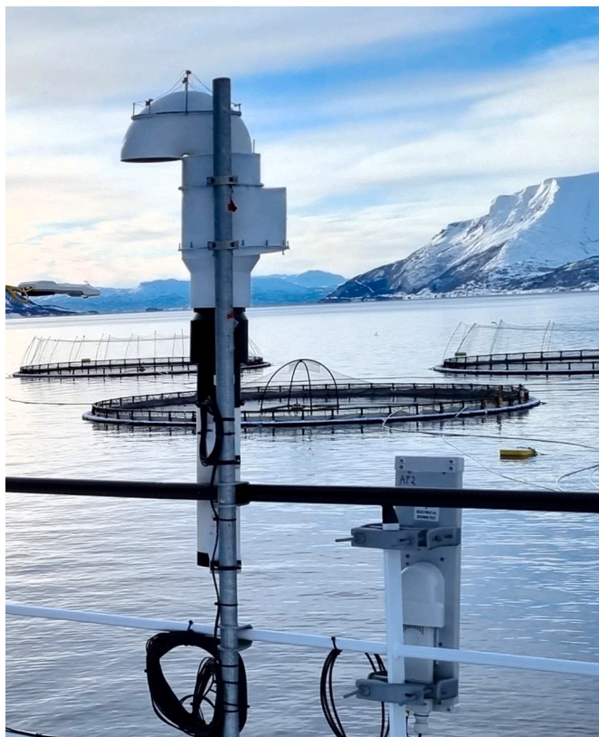
Fig. 27. SPRICE collector installed on top of the feed barge, facing the west-southwest (WSW) direction.
