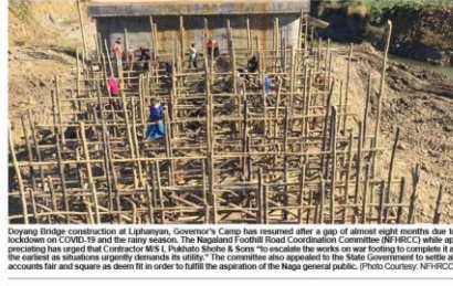
Doyang Bridge construction at Liphayim, Governor's Camp has resumed after a gap of almost eight months due to lockdown on COVID-19 and the rainy season. The Nagaland Road Coordination Committee (NRCC) while appreciating has urged that Contractor M/S. I. Pathak Shree & Sons "to escalate the works on war footing to complete it at the earliest as situations utterly demands its utility." The Committee also appealed to the State Government to settle all accounts fair and square as deemed fit in order to fulfil the aspiration of the Naga general public. (Photo Courtesy: NRCC)
