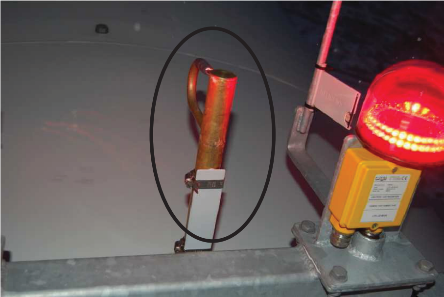
Figure 3.10: HoloOptics sensor, inside the ring, as installed on the light boom.
