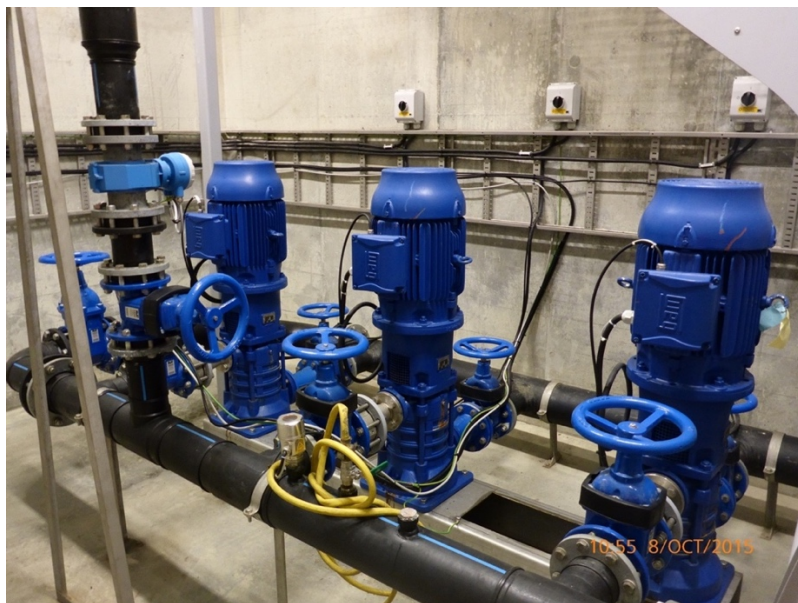
Figur 10 Pumperom i Ryatunnelen (Aas-Pettersen, 2015)
